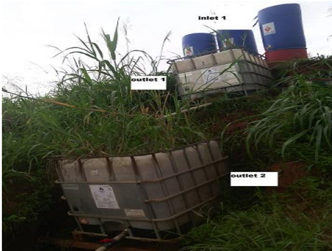
Figure 7: Subsurface vertical-flow reed beds treatment system.
