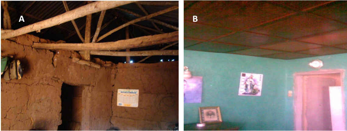
Figure 5. A) Habitat showing a lot of space between the rough wall and the roof with several cracks in the wall (Dangbo); B) habitat with a ceiling and smooth wall without cracks or spaces (Dangbo).
