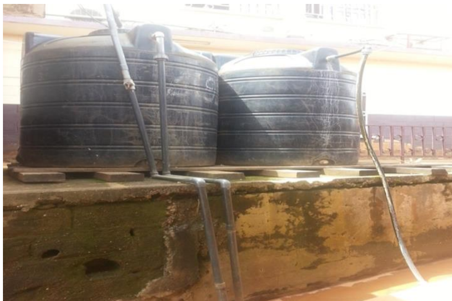
Fig 32: Tanks for potable water storage
