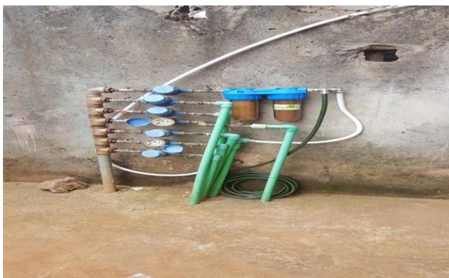
Fig 28: Filtered water from the meter
