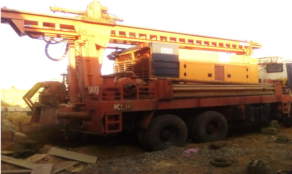
Picture 1: Deployment of Heavy Machinery Equipment for the Construction of a Borehole to supply water for a Hotel and a Supermarket
