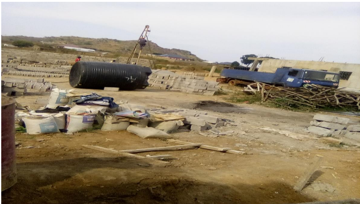
Picture 8: Installation of Equipment for the Construction of a Borehole for a Household
