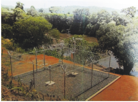
FIGURE 3: Equipment of the station of Kadey with Batouri in automatic station.
