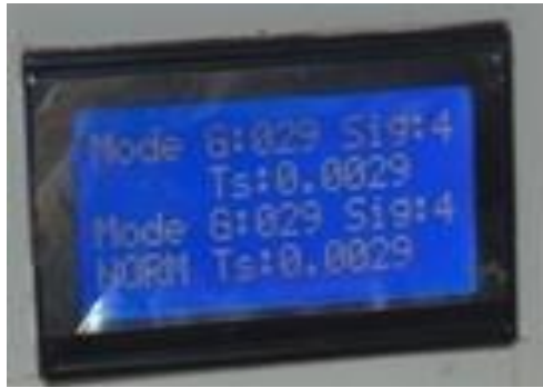
Figure 3.34 Screen of the generator.
